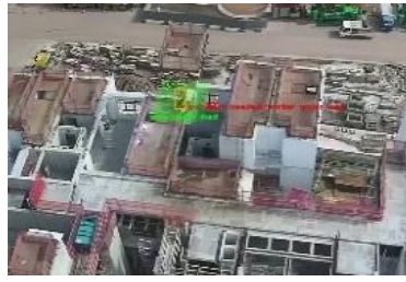
Worker under lifted load
